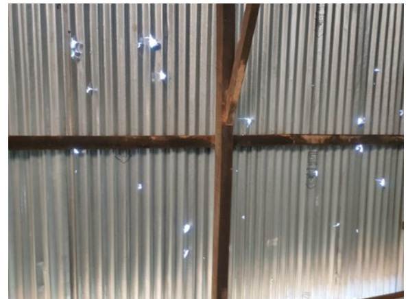
Damage caused to houses due heavy hailstones
